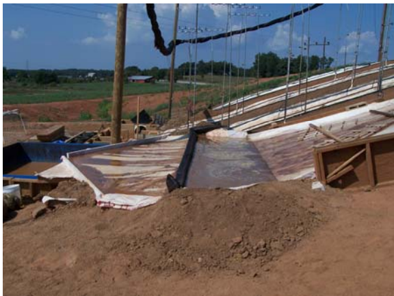
Figure 4. Seepage (left) and Ponding (right) as Wattle Intercepts Runoff
